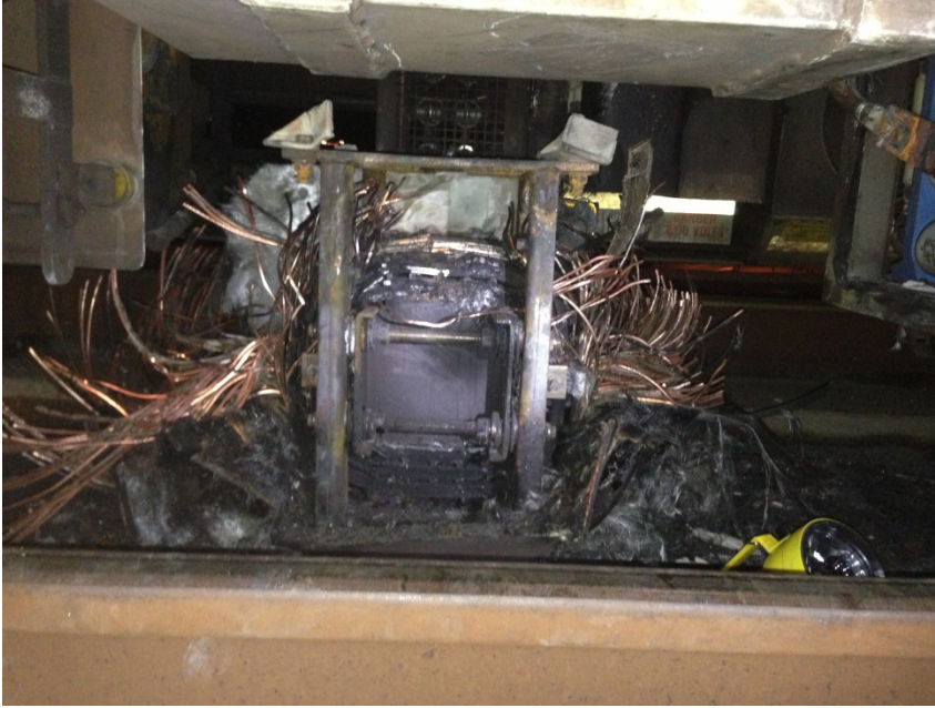
Burnt semi-conductor box prior to removal from platform
