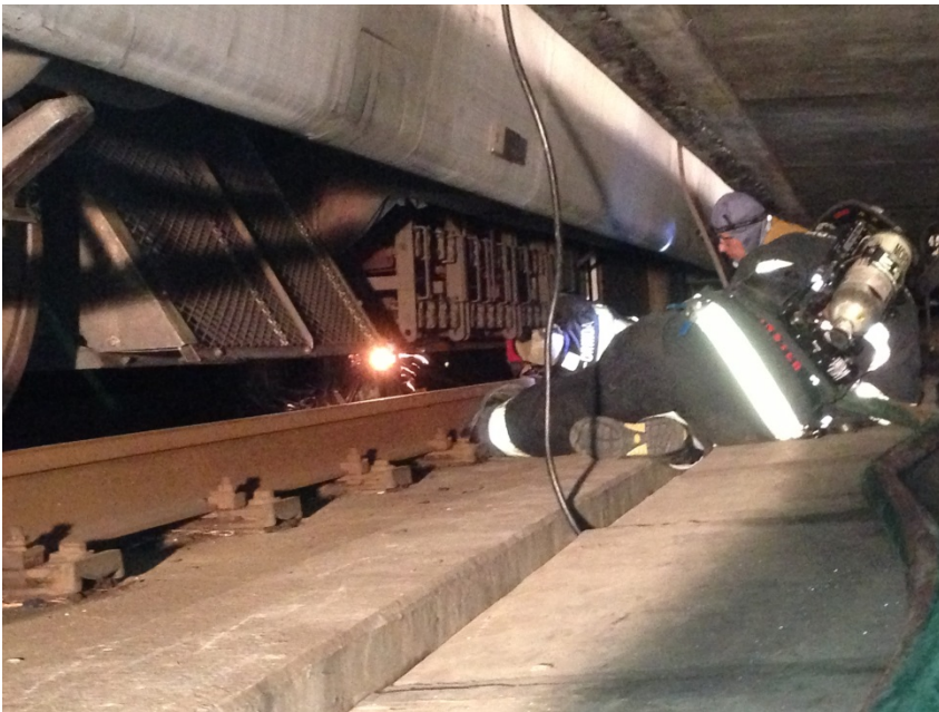
Moraga-Orinda Fire District Firefighter and BART employees cutting the semi-conductor box with the torch so box could be removed from underneath train
