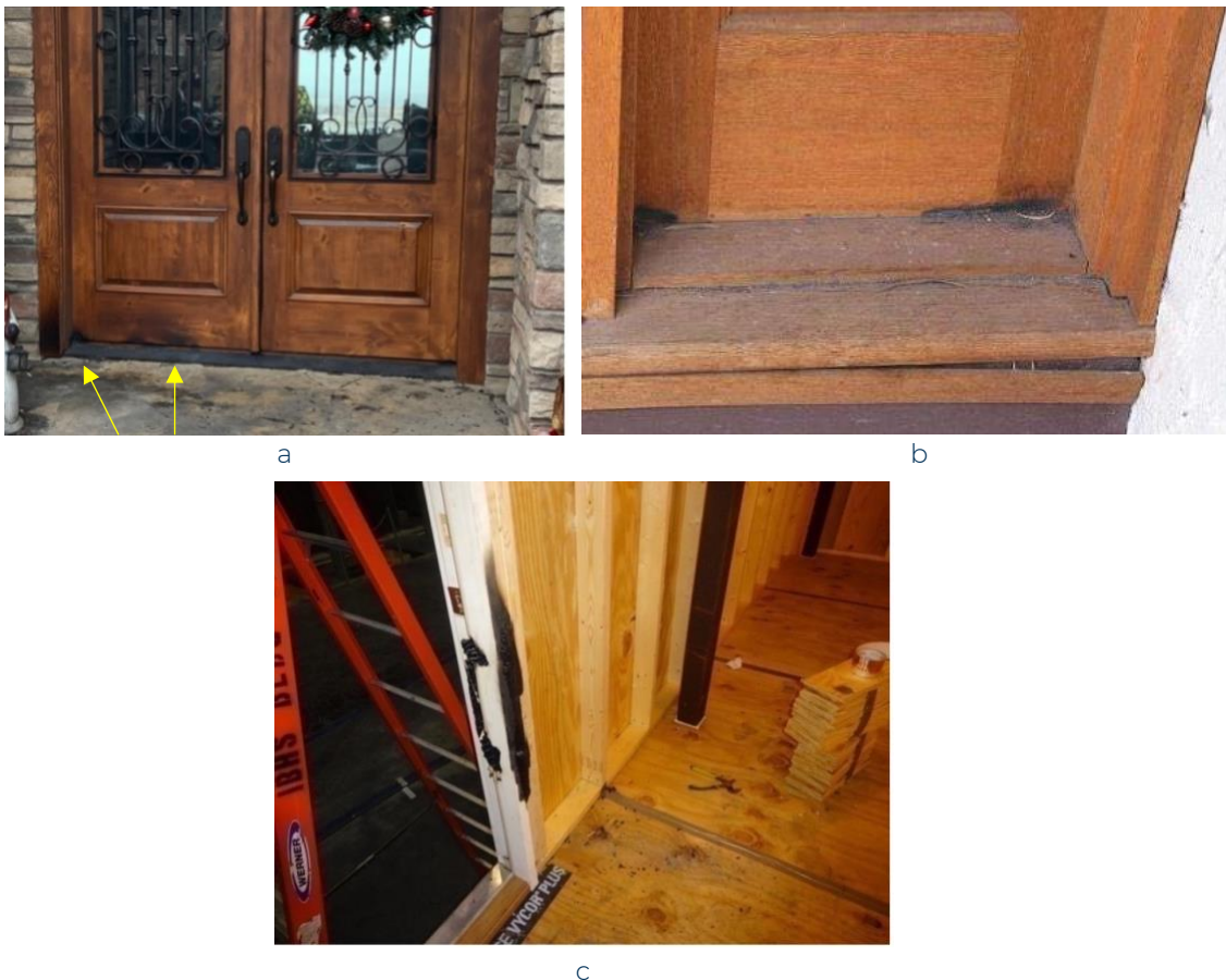
Figure 14. (a) Post-Marshall Fire (2021) investigation in Boulder County, Colorado, showing evidence of ignition from an accumulation of embers and debris at the base of the door; (b) Embers charred the threshold during the Victorian Bushfire (2009) in Australia ( Leonard, 2009 ), used with permission; (c) Embers ignite the door jamb at the IBHS Research Center.
