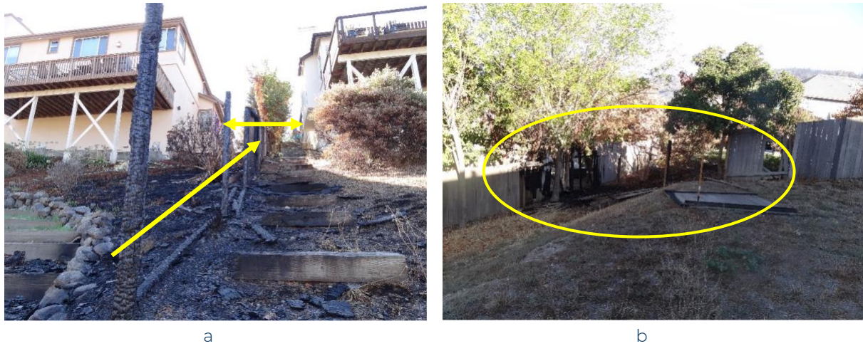
Figure 10. In the Glass Fire (2020) in Napa and Sonoma Counties, California, (a) a combustibility fence provided a pathway for fire to spread uphill and damage both homes during fire, and (b) a wood fence spread fire and led to a cascade of damage (defended).
